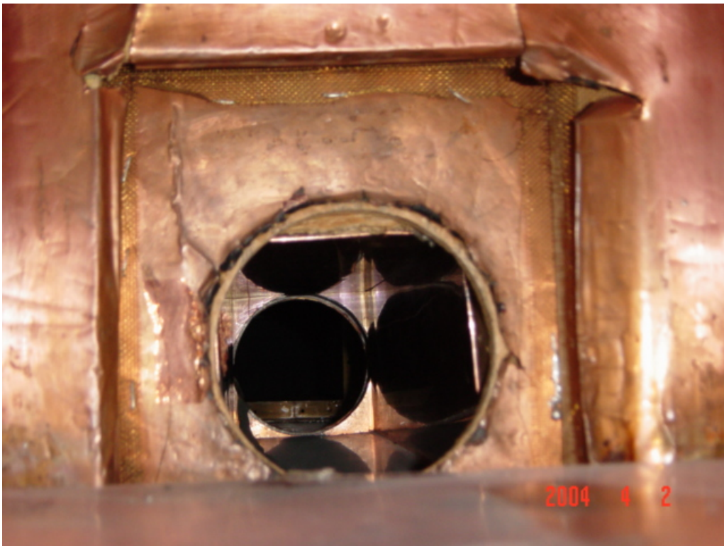
Figure - 5: Room 11P Waveguide Opening (Monitor Room)
