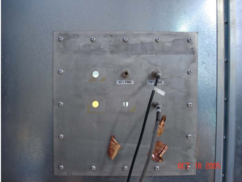
Figure – 4: Monitor room plate
