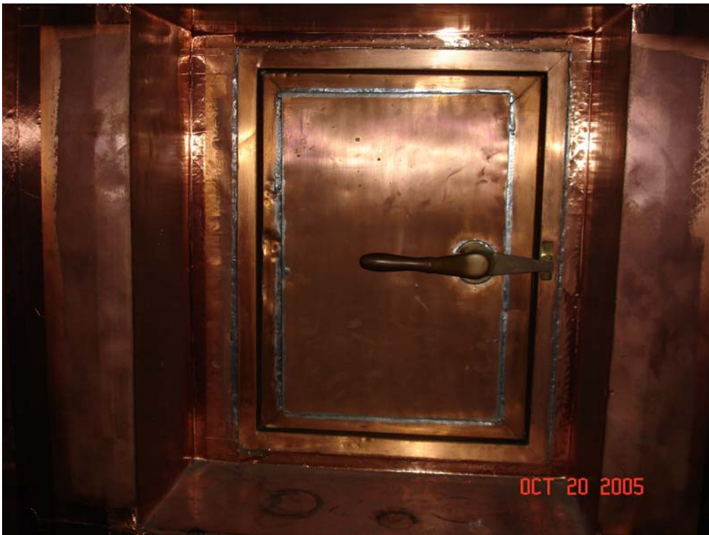
Figure – 10: Access Hatch
