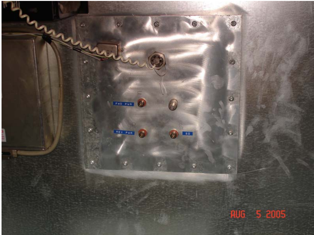
Figure – 11: Room 24P (Monitor Room) Outer Mounting Plate Plate #4
