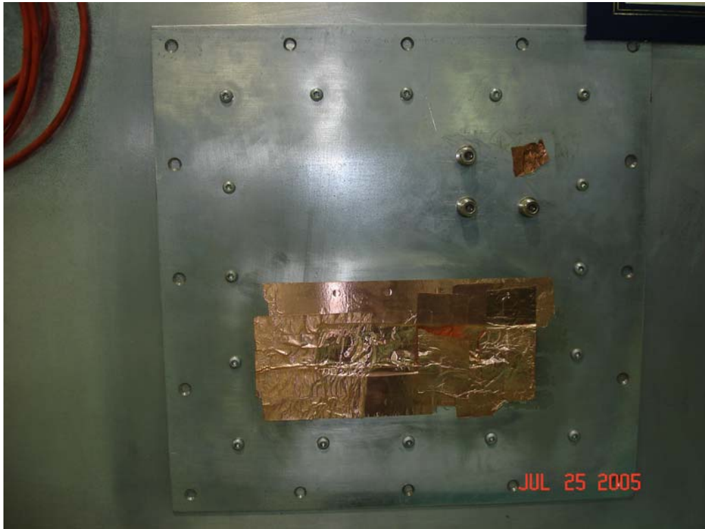
Figure - 6: Room 24S (Test Room) Outer Mounting Plate (View from outside chamber) Plate #2
