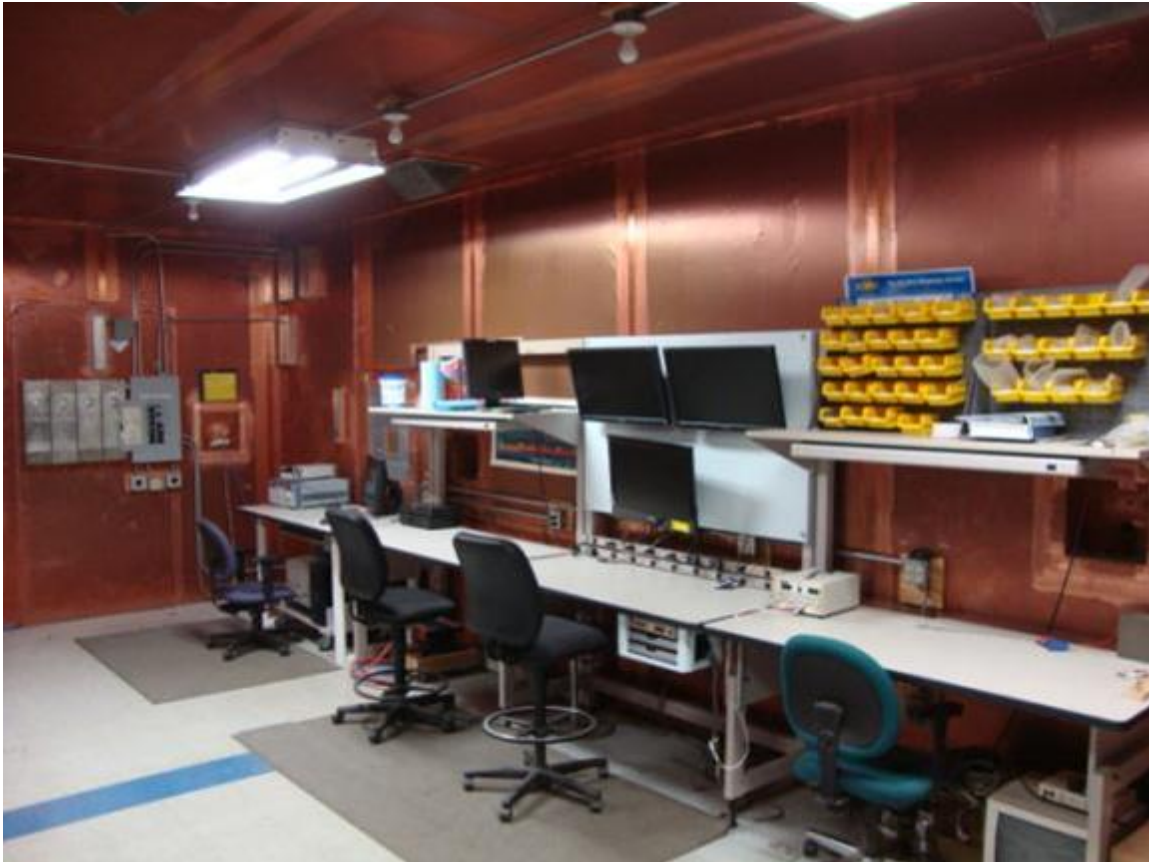
Figure – 3: Room 22P (Monitor Room)
