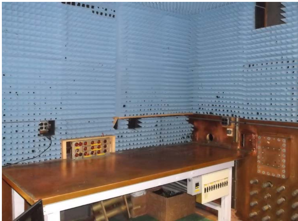
Figure - 2: Room 19P (Monitor Room)
