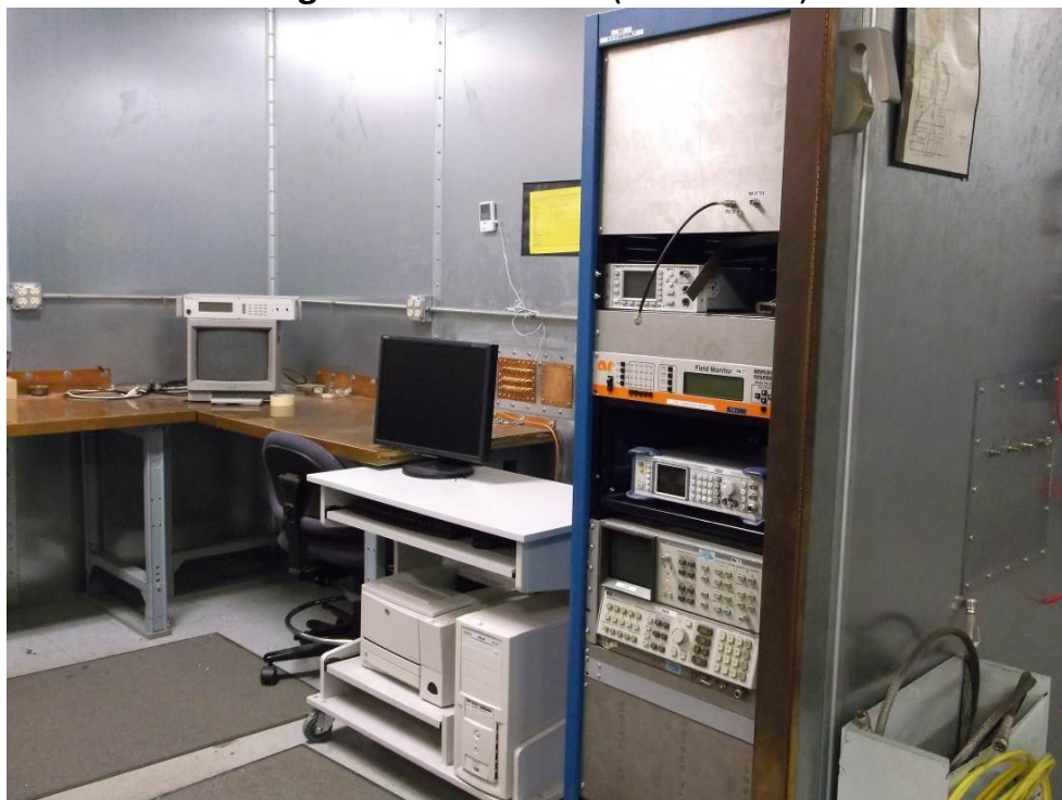
Figure-2: Room 27P (Monitor Room)
