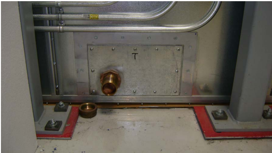
Figure – 9: Test Chamber Access plate
