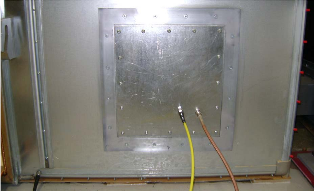
Figure – 6: Monitor room plate
