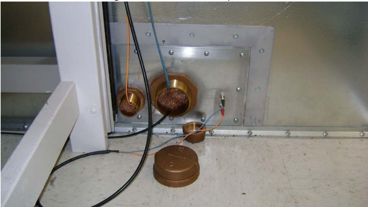
Figure – 7: Control room plate
