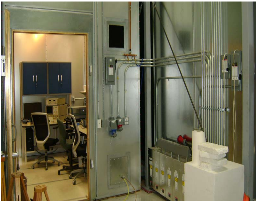
Figure – 4: Room 29P (Monitor Room)
