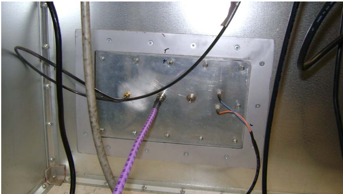
Figure – 8: Control room Receiver plate & Antenna Mast controller
