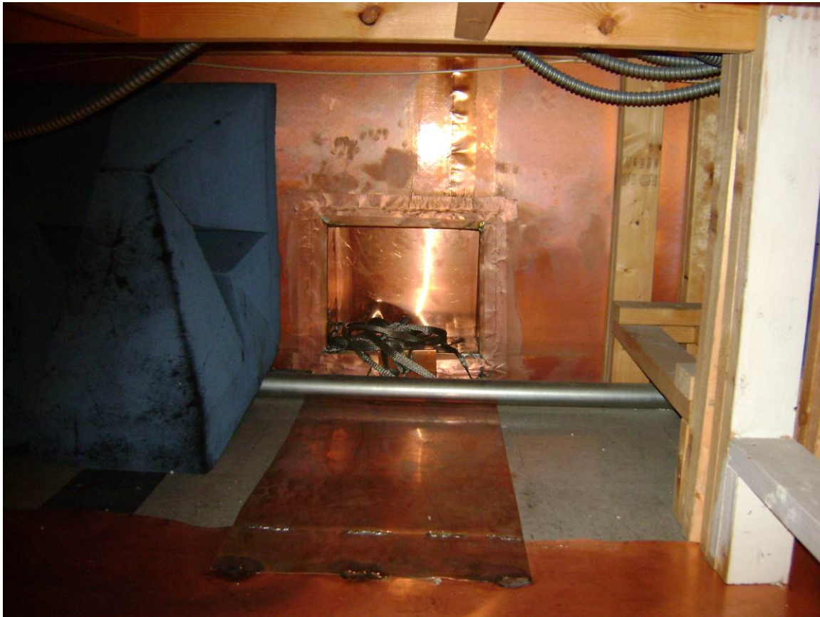
Figure – 8: Room 23M panel below ground plane to 23L under the ground plane. 13 ¾ inch by 11 ½ inch high opening (Plate #3)
